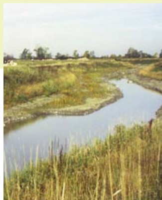
Riffle and pool structures were strategically placed into the south branch of the South Nation River municipal drain in Dundas. The work was completed as part of the engineer's report, in hopes of providing fish habitat.
