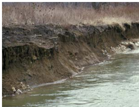
Bank erosion from streamflow.
