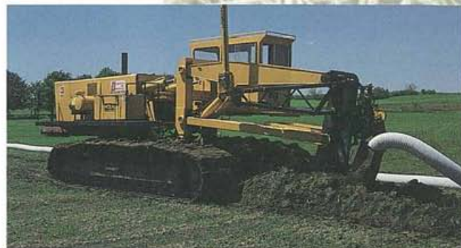
Drainage is an important component in a mulch till system. Make sure wet fields are tiled first before starting mulch tillage.
