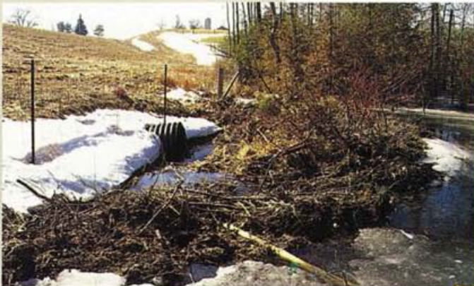
Beaver dams can cause significant financial loss due to flooding of farm fields and roads.
