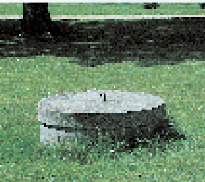
Every year you should check that the sanitary seal and well cap are secure and watertight.
