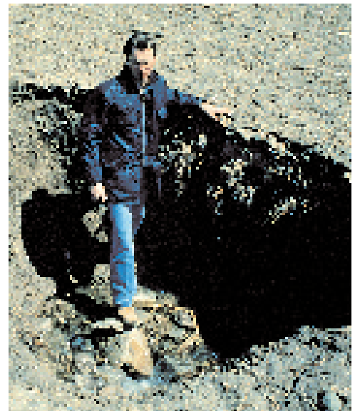
A tile blowout or wash-in indicates immediate attention is needed to repair the tile drain.
