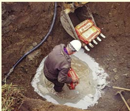
A final plug of bentonite was created to prevent any movement of liquid down the old casing.
