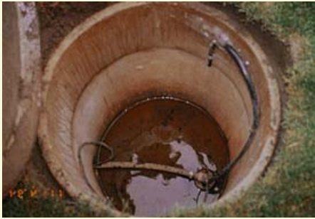
Prior condition: water and debris collected in pit, with risk of moving down drilled well casing.
