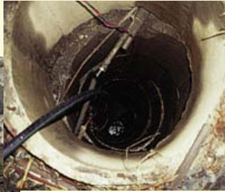
Prior condition: old dug well had been replaced with a drilled well nearby, and old well presented a risk to groundwater quality and personal safety.
