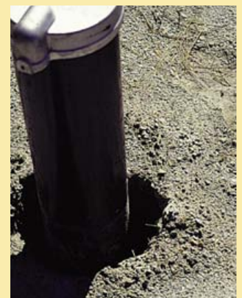
If not sealed, the annular space around this drilled casing could convey contaminated surface water directly into the aquifer.
