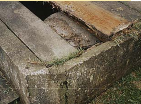
Wooden planks covering well pits are not watertight and can rot, presenting a safety hazard.
