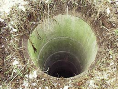
Prior condition: bored well had not been used for decades, and the only protection was a steel mesh grate. The situation presented a risk to groundwater quality and personal safety.
