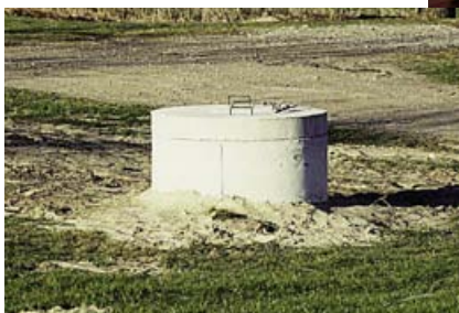
Using clean clay, mound the ground around the outside of the well casing.
