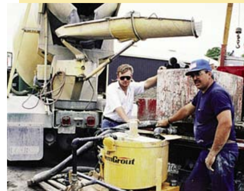
Contractors grout the annular space around the outside of the casing of a newly constructed well.
