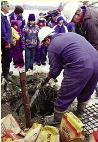
Water was added to activate the bentonite clay. Clean clay soil was added above the bentonite plug to within 3 metres (10 ft.) of the ground surface.
