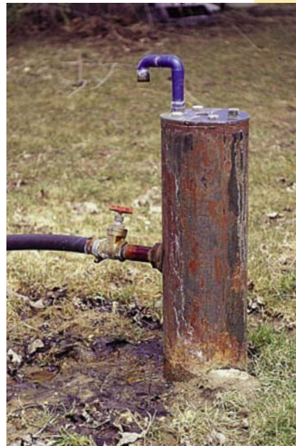
The relief valve on the casing offers some control of this flowing well. However, by itself it's not considered an acceptable construction practice.
