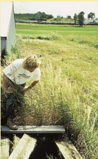
This is an unused well in very poor condition. Until it is properly plugged, it poses a threat to groundwater quality, and the safety of humans, livestock and wildlife.
