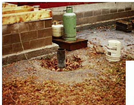
This is a problem situation: there is no watertight cap, and settling around the casing suggests a poor annular seal.
