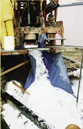
Redeveloping wells involves clearing encrustation from the well screen, or removing plugs in the formation around the screen.
