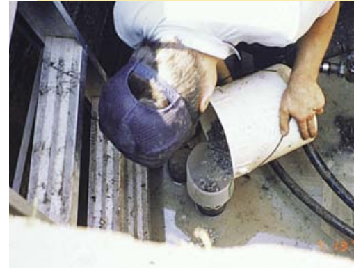
Pouring dry bentonite down an unused drilled well casing may not form an effective plug. The material can stick or form a bridge in the casing, leaving gaps in the seal.
