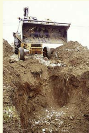
The hole was filled with clean clay soil, mounded to direct surface flows away, and seeded. A Water Well Record describing the procedure was completed and filed with the authorities. Total material and labour costs were $695.*
