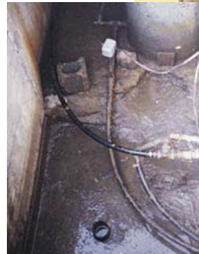
The abandoned drilled well in this pit has not been properly plugged. The situation invites serious contamination.
