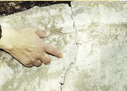
Visible cracks in the casing should be sealed promptly.
