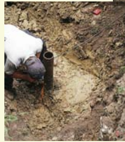
Steel casing was trimmed down and an adapter plate welded on to accept casing extension.
