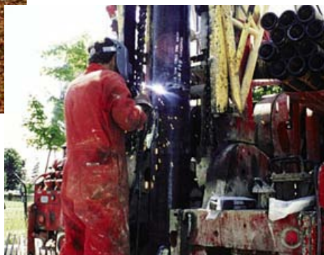
Joints between sections of steel casing are welded as they are lowered into the well.
