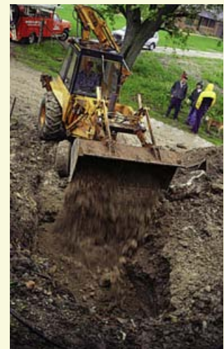
Hole was filled in with clay soil, mounded to direct away surface flows, and seeded. Total cost for materials and labour provided by a licensed contractor was approximately $600*. A Water Well Record describing the procedure was then filed with the proper authorities.
