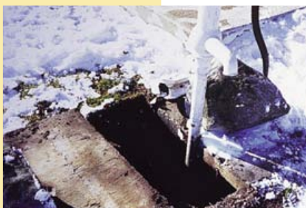
Abandoned wells should never be used as disposal sites for roof water, septic wastes or any other organic debris.
