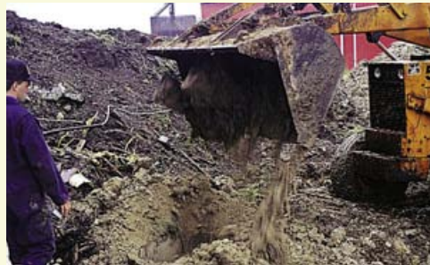
Clean clay fill was added to within 3 metres (10 ft.) of the ground surface.
