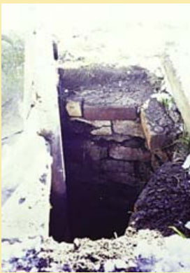
With or without a proper cover, the brick lining on this old well can present problems.
