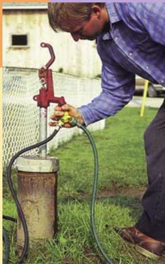
This drilled well casing has had a frost-free hydrant added with a backflow preventer.
