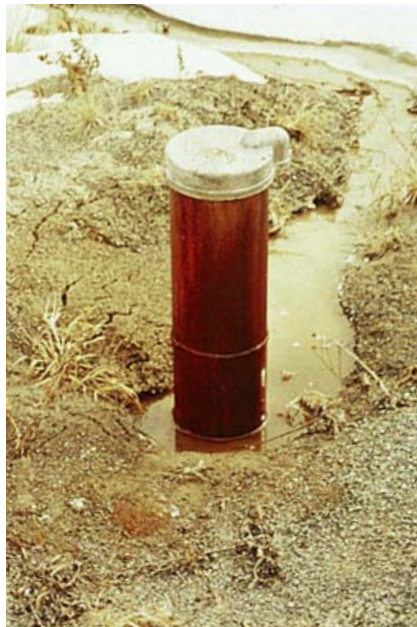
No flow-control device was included in the installation of this artesian well. The pressure has resulted in water flowing up the outside of the casing to the surface. This is poor workmanship.
