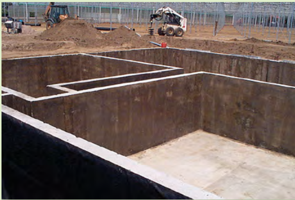
This below-ground reservoir can store fresh water, nutrient feedwater, or disinfected or treated leached nutrient feedwater.
